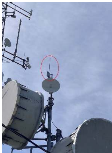
Figure 5: A Crypto rig (proof-of-coverage) illegally placed on tower site.
